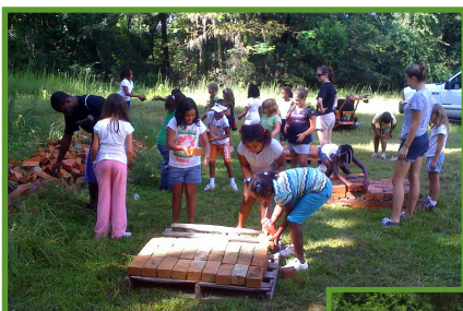
Girl's Place campers clean and stack bricks at the Historic Rochelle Church stabilization project.
